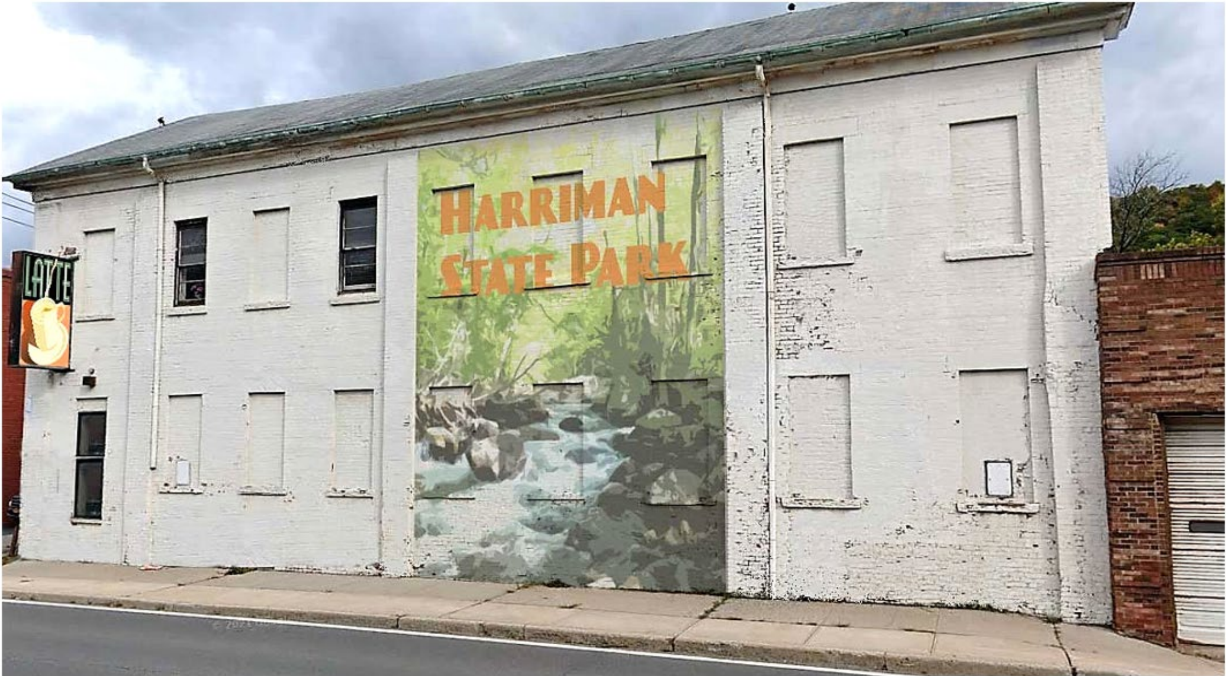
Figure 9: Mural simulation #2-image of regional interest-Harriman State Park. (Photo courtesy of Google Streetview)
